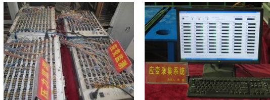
Fig. 11. Strain and pressure test system
