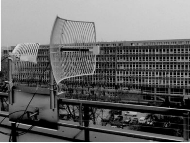
Fig. 1. SAR antennas at ISE PW "terrace SAR" lab.
