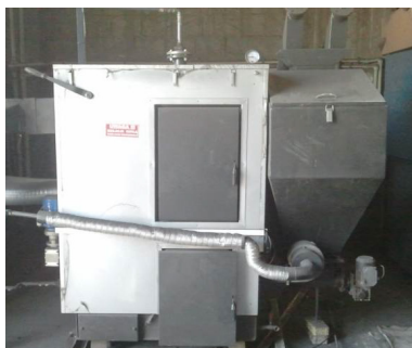
Fig. 1. Prototype of the experimental coal-fired installation built within the scope of the project
