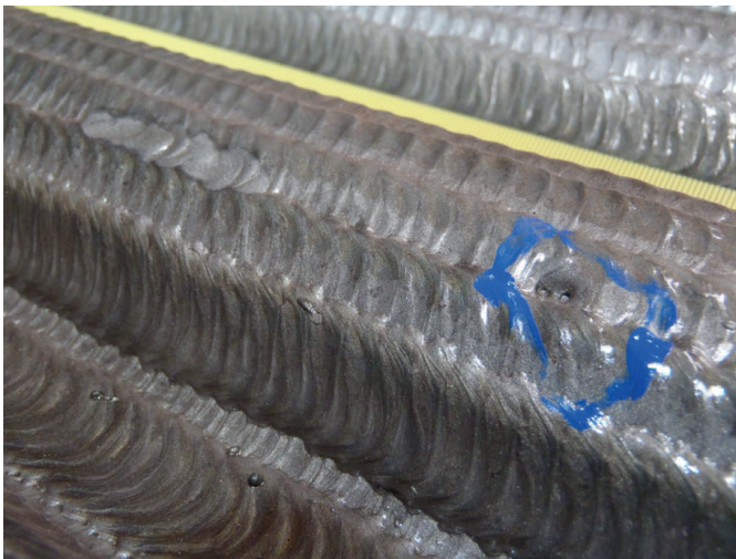
Fig. 1. Piping in the surfacing weld
