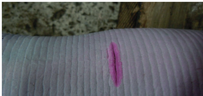
Fig. 16. An indication of the crack after PT on the singular pipe spirally surfaced by welding
