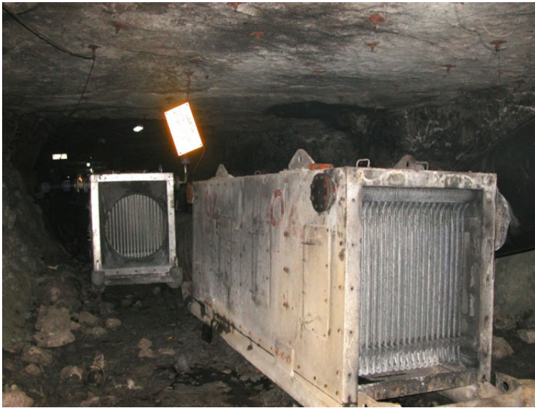
Fig. 4. GCP 350 mine air cooler
