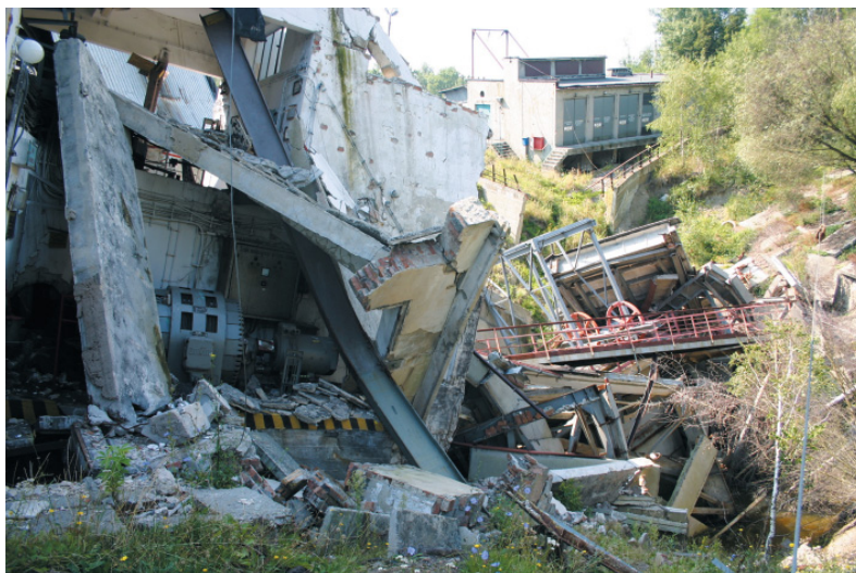
Fig. 1. Construction failure on a shaft object caused by the lack of corrective action
