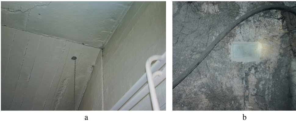
Fig. 3. Recorded damage a) displacement of ventilation head, b) view of the installed seal
